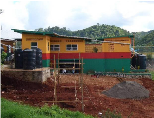
Water Tanks, Kitchen Classroom # 2 & Toilets
