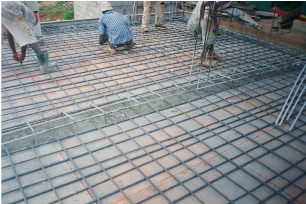
Classroom Floor showing poured center beam (with supporting column in basement beneath)
