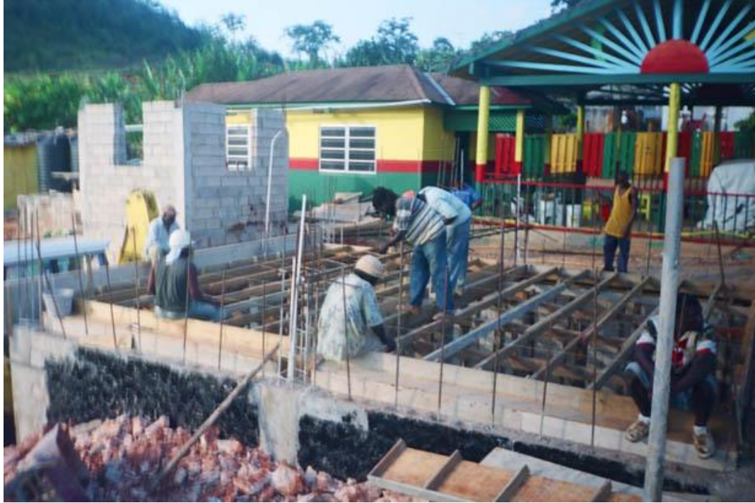
Waterproof Basement with plaster & pitch. Form and pour for concrete beams & floor for classroom
